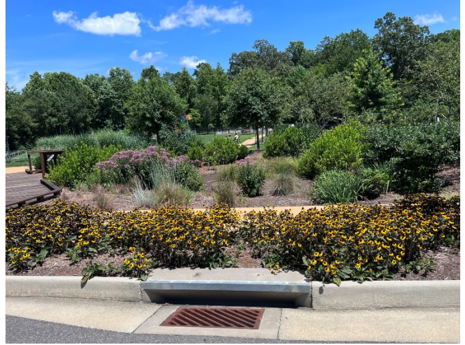
One of five Stormwater Swales planted with Native Plants
